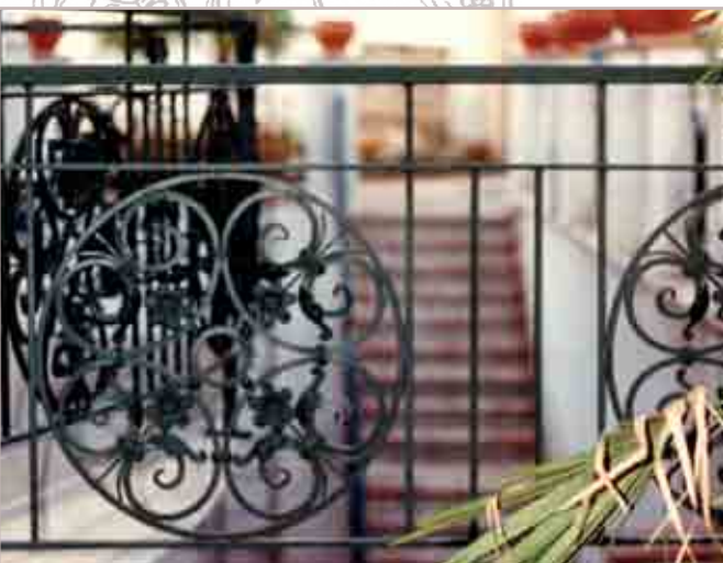
Dettaglio parapetto esterno / Detail of the outdoor balconies Detalle barandilla externa / Détail garde-corps extérieur
